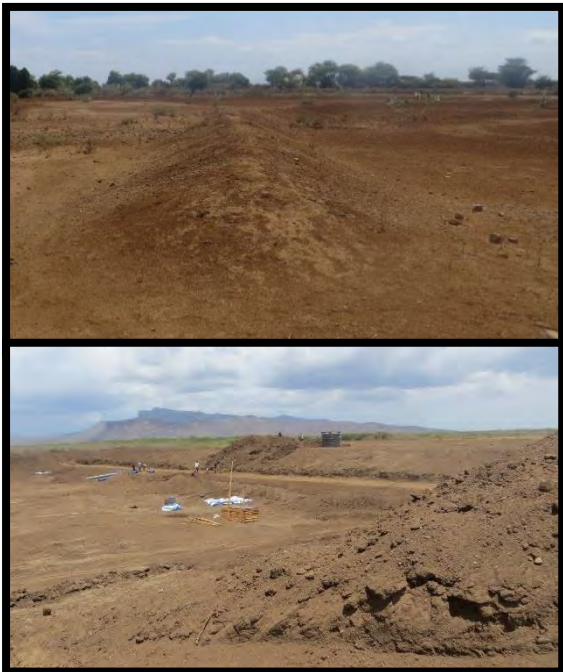
Image 16: Above: Trapezoidal bunds at the border of a dry river bed, below: Construction of water reservoir
